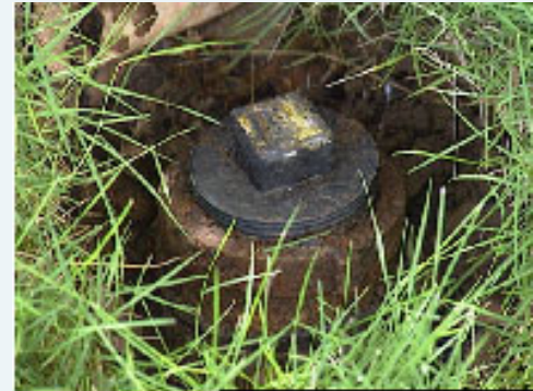
Typical sewer cleanout with properly installed plug.
